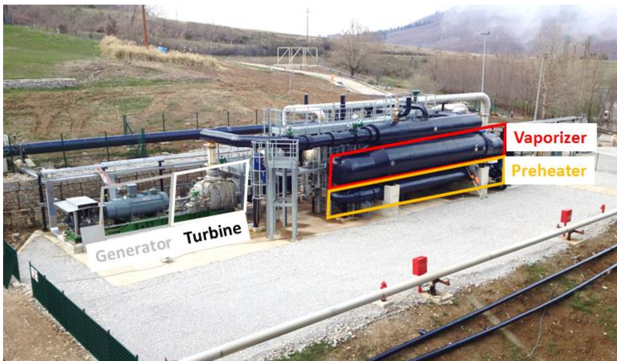
Figure 3. Bagnore binary power plant.
